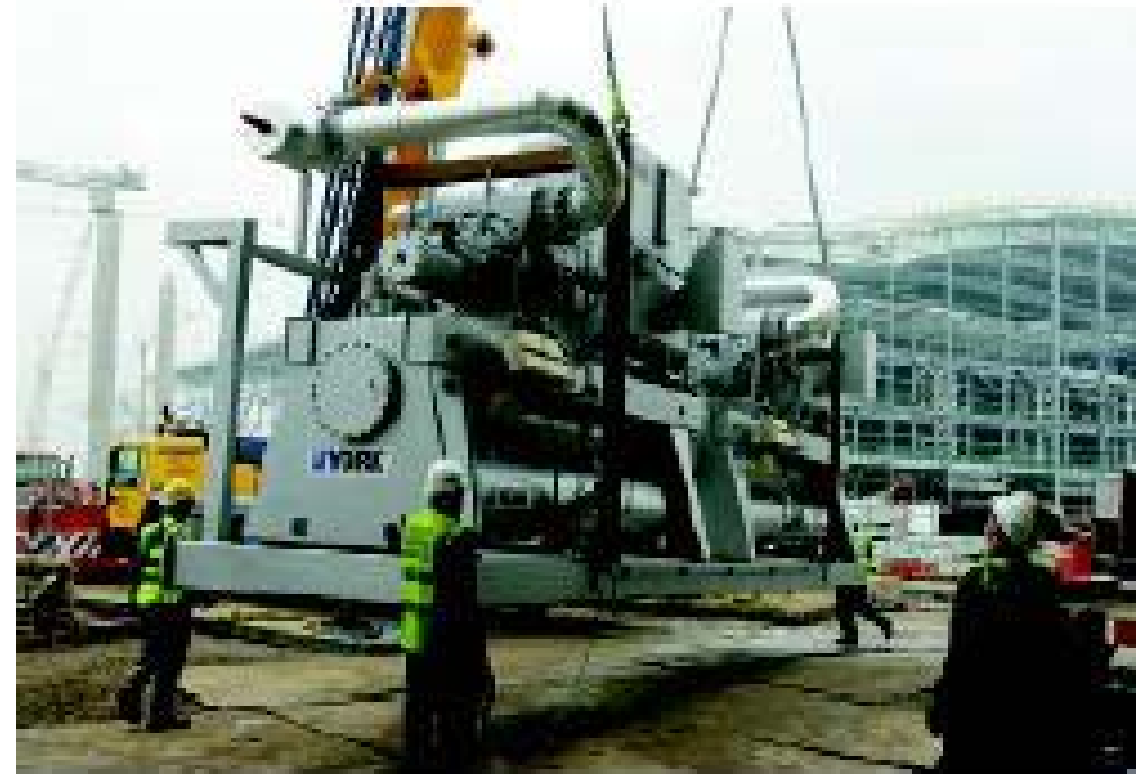
One of four 6.6 MW ammonia chillers arrives at Heathrow Airport's Terminal 5 project.
