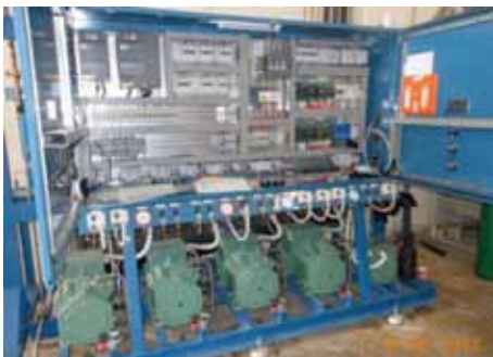
Fig. 2 The CO 2 compressor rack
