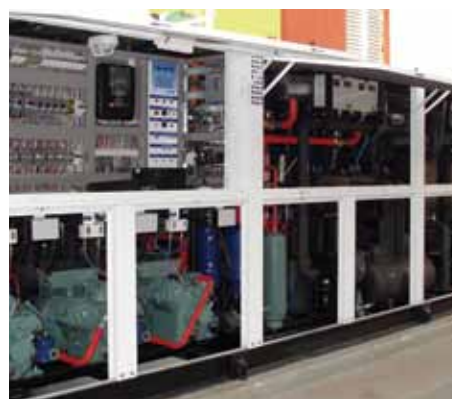
Fig. 5 The refrigeration system
